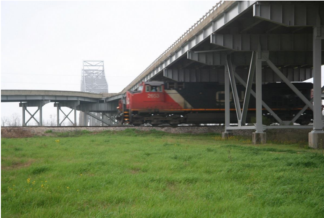
Condition Photo 19: Easterly approach span over the CNRR, with Y-split in background.
