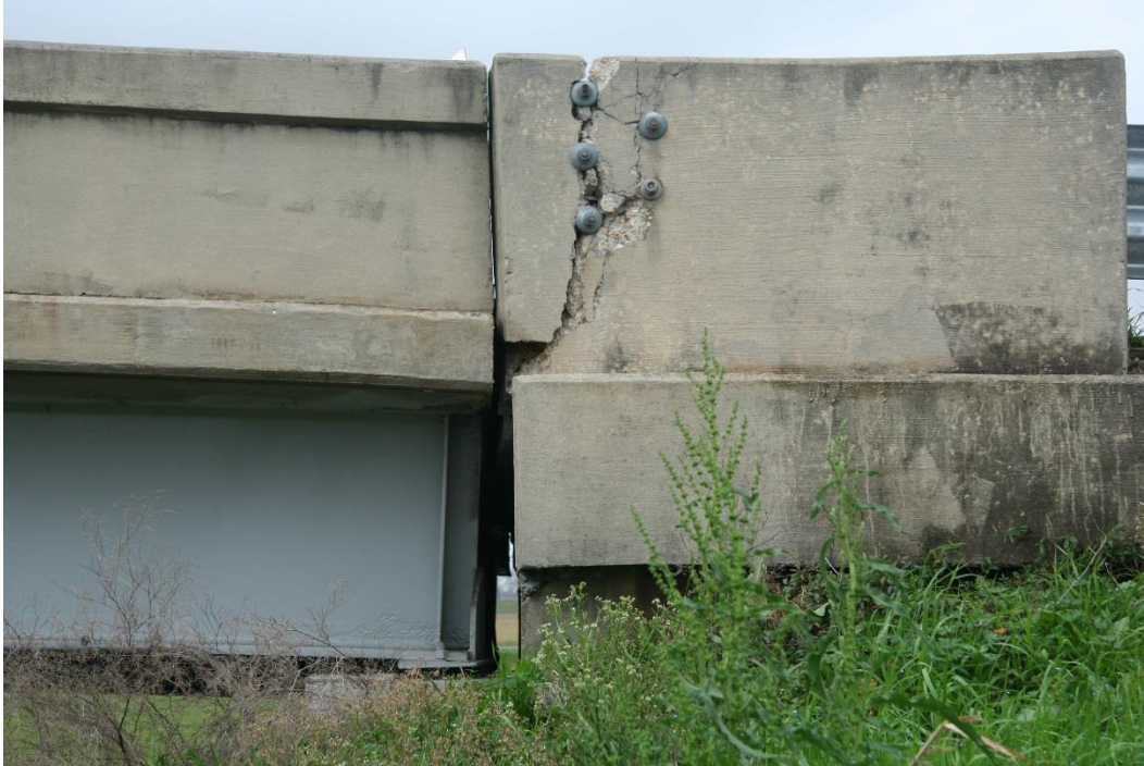
Condition Photo 17: Damaged barrier railing attachment at end of northerly Y-ramp
