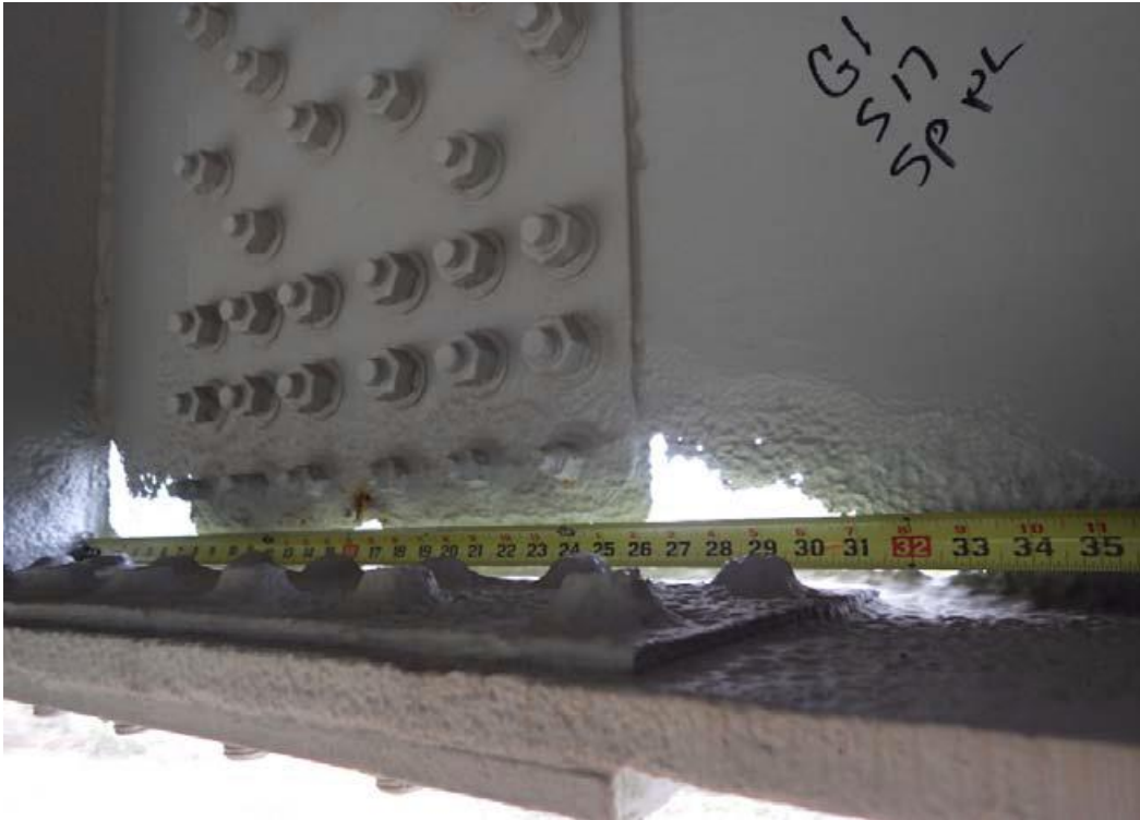
Condition Photo 23: West approach span 17, girder 1 has 100% section loss in the web near bottom flange at the splice plate. Photo courtesy of the LADOTD from inspection performed March 7, 2016.
