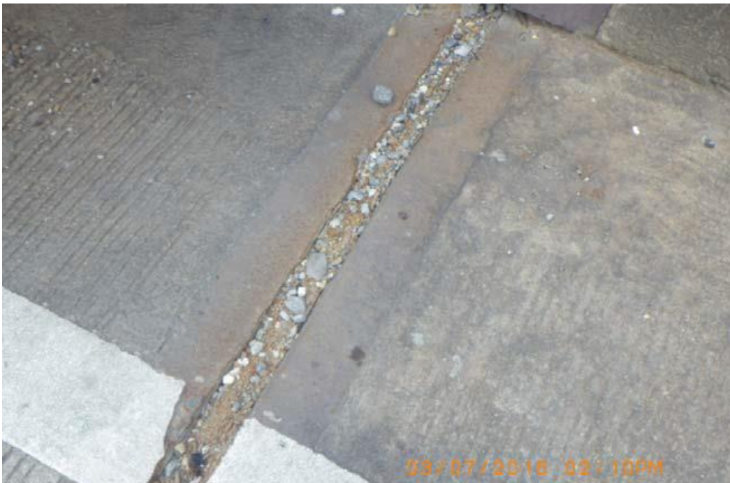
Condition Photo 24: Compression seals have a heavy accumulation of rocks and debris throughout the structure. Photo courtesy of the LADOTD from inspection performed March 7, 2016.
