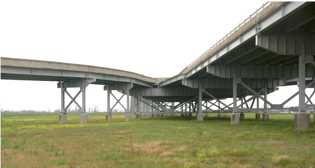
Historic Fabric Photo 2: Y-shaped approach ramp spans at the easterly end of the bridge, including floor system and braced steel column towers.
