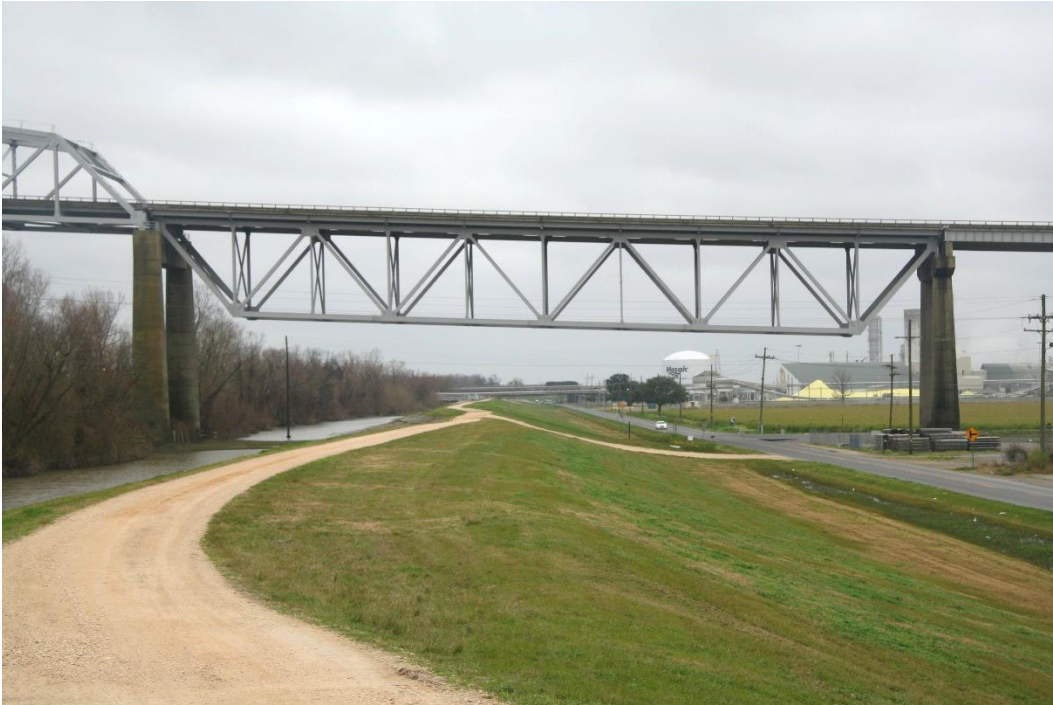
Historic Fabric Photo 1: Deck truss approach span to the west of the main Warren through truss spans, spanning LA 18 and the westerly levee of the Mississippi River, and approach piers.
