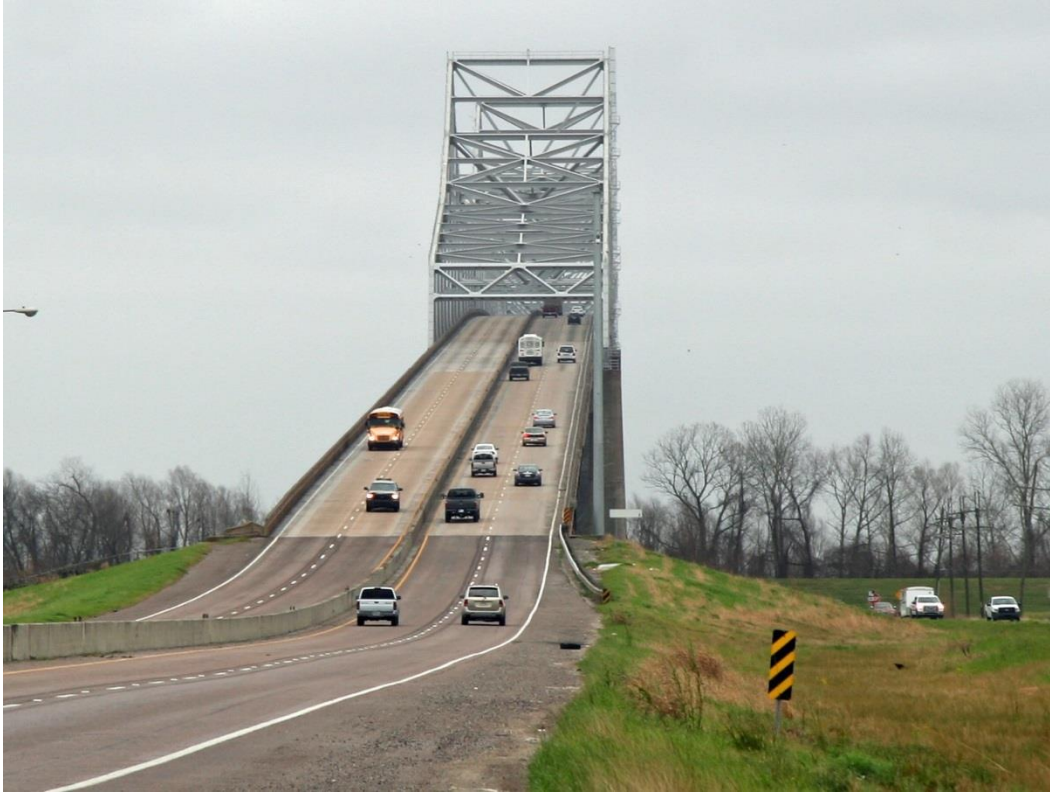
Condition Photo 9: View from west end of bridge looking east toward the bridge.
