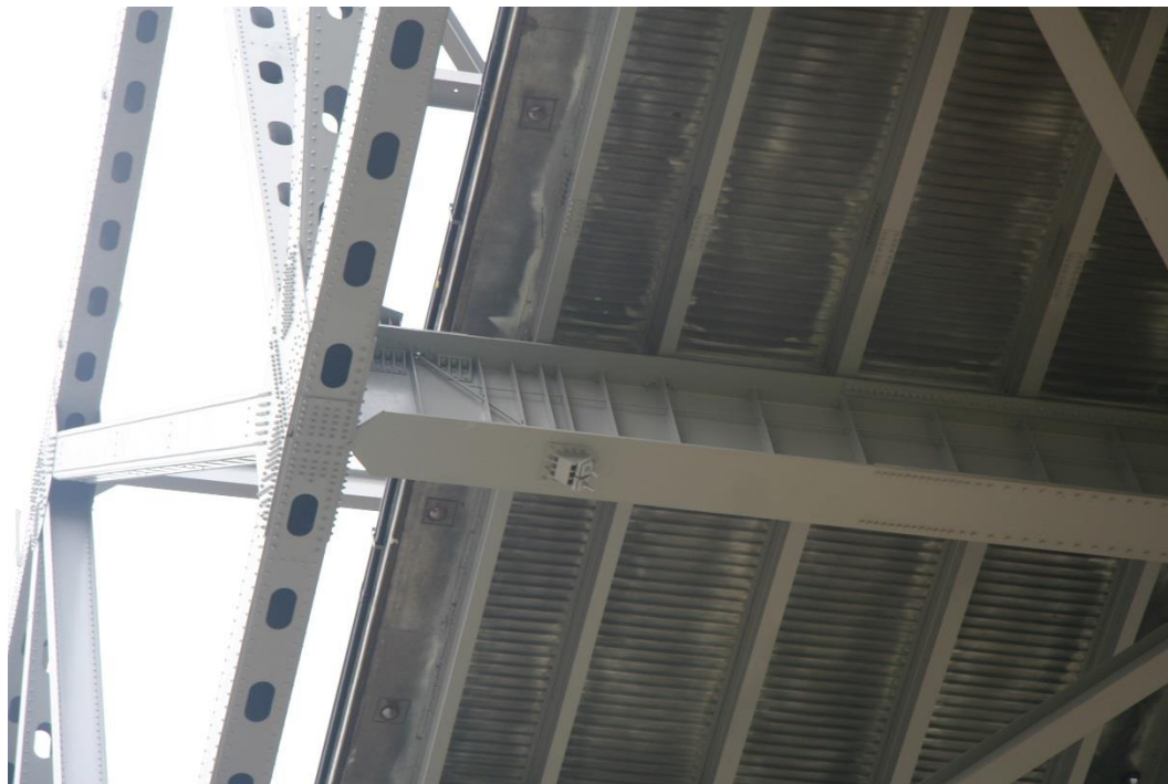
Condition Photo 14: Underside of truss span showing floor beams, stringers and deck system.
