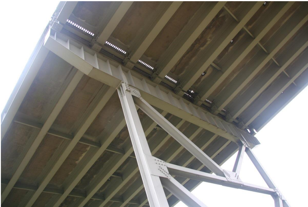
Condition Photo 4: Westerly approach spans with finger-type deck expansion joint at Bent 20.
