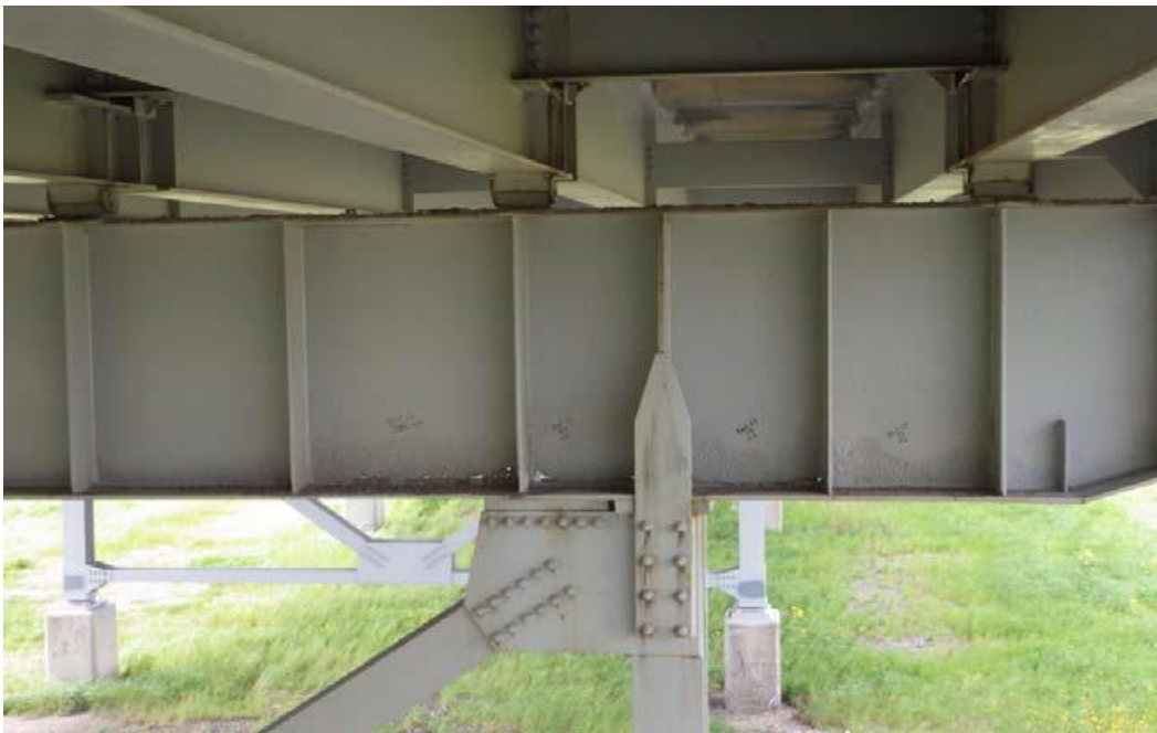
Condition Photo 22: Bent 54 cap has 100% section loss in web, which is typical for bent top girder; rust stains noted to the tops of the floorbeams. Photo courtesy of the LADOTD from inspection performed March 7, 2016.
