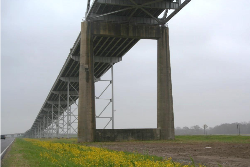
Historic Fabric Photo 3: Approach spans to the east of the main Warren through truss spans including floor system, braced steel column towers, and approach piers.
