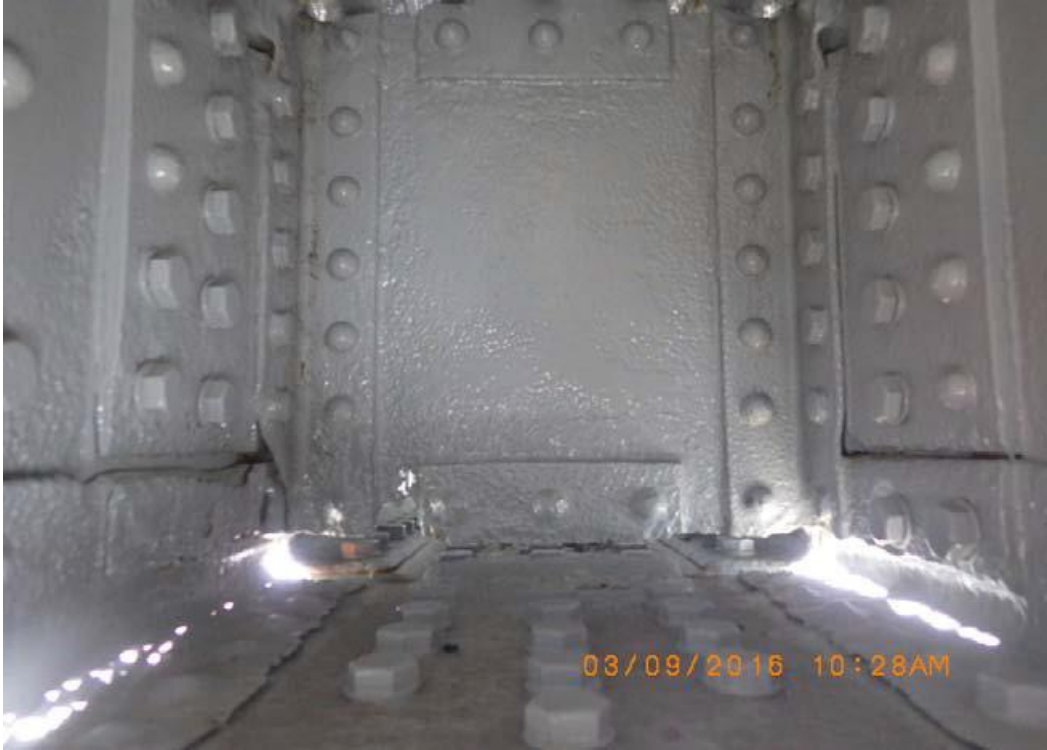
Condition Photo 21: View of heavy section loss to the inside of the lower chord at joint L19. Photo courtesy of the LADOTD from inspection performed March 7, 2016.
