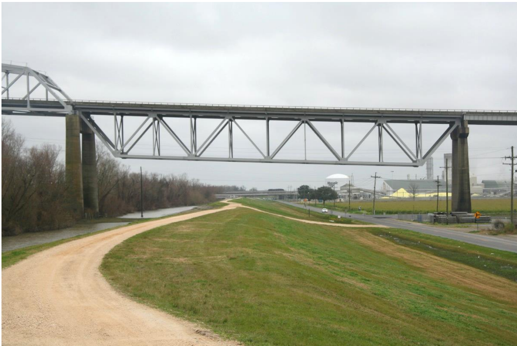
Condition Photo 8: Deck truss span 18 over LA 18 and west levee.
